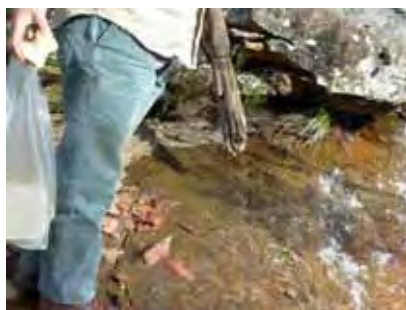
The main impacts on faunal values in the site are associated with longwall mining, such as streambed cracking. DECC
