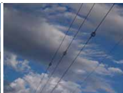
Powerlines crossing Port Hacking require bird strike mitigation devices such as these. M. Schulz
